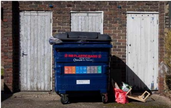
Inadequate refuse stores
