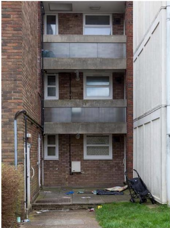
Lack of legibility - where is the front door?
